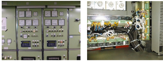
Fig. 1: Monitoring and control of automation subsystems in large scale systems may comprise 20.000 of I/O-points. Photo: Kongsberg Norcontrol (first; Berge Nord, second & third; Main switchboard outside & inside)
